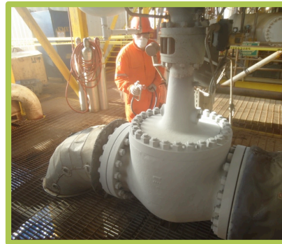
Steam System Insulation Pemex - Offshore Mexico
